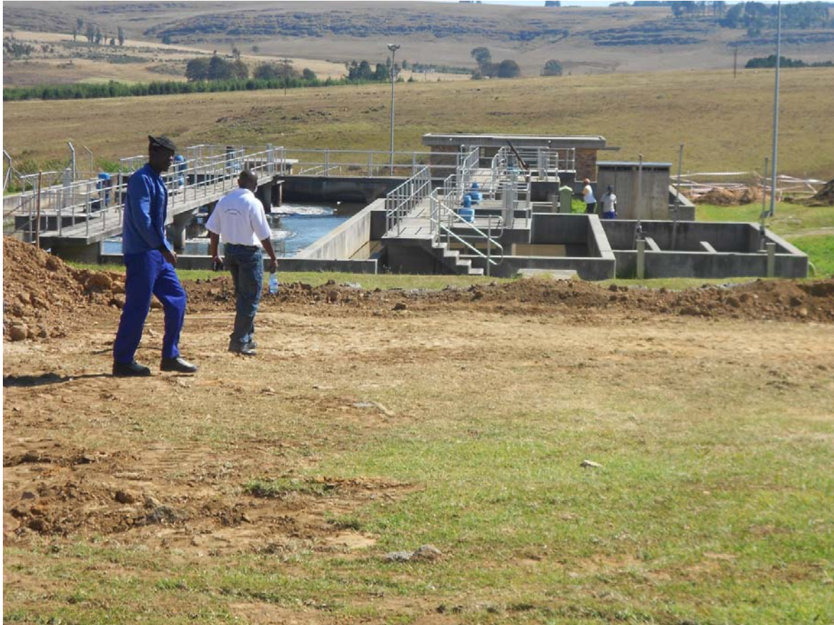
FIGURE1: UPGRADING OF WASTE WATER TREATMENT WORKS IN DULLSTROOM
